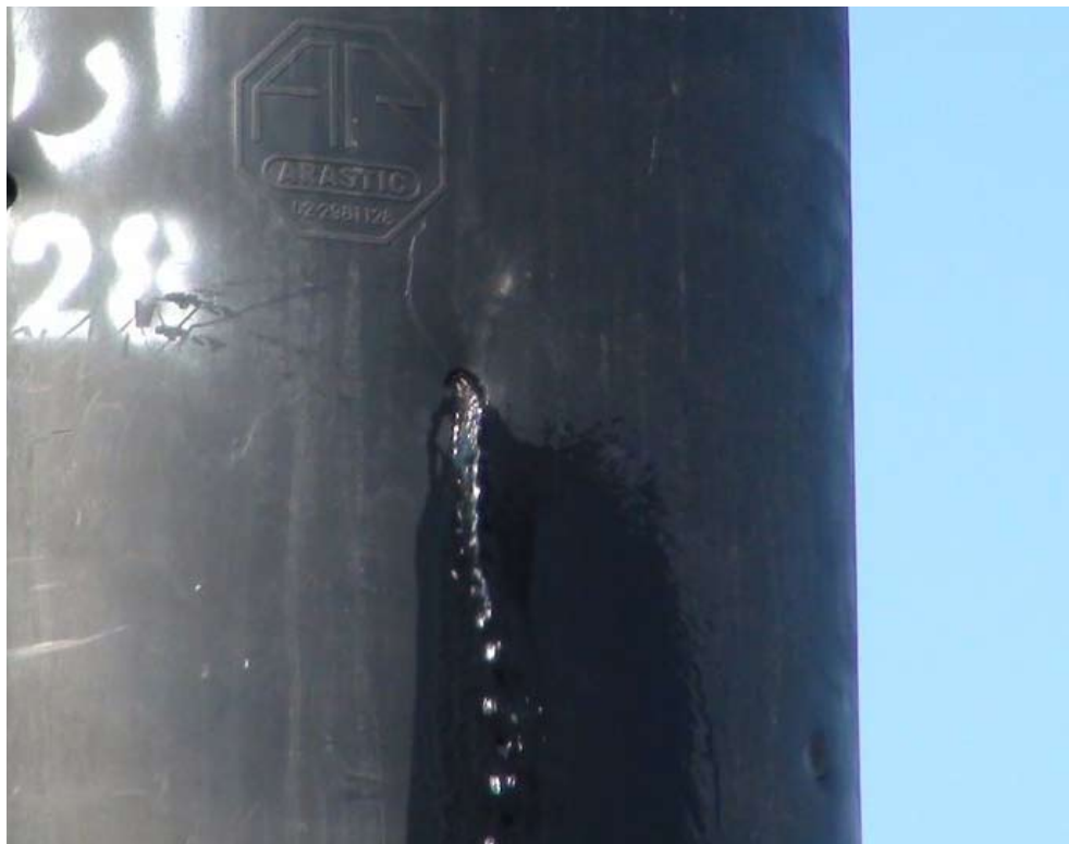
Water tank with a hole in it, a result of being struck by a tear-gas canister (Sarit Michaeli, B'Tselem, 24 June 2011)
