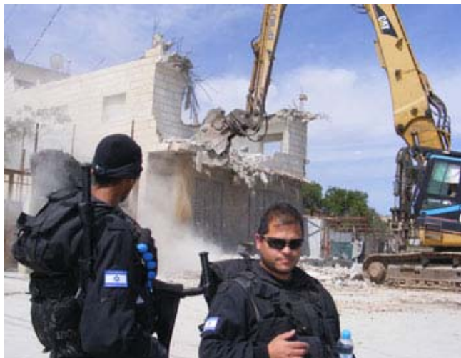
Demolition of the Dwayat family's house, East Jerusalem. Photo: Kareem Jubran, B'Tselem, 7 April 2009.
